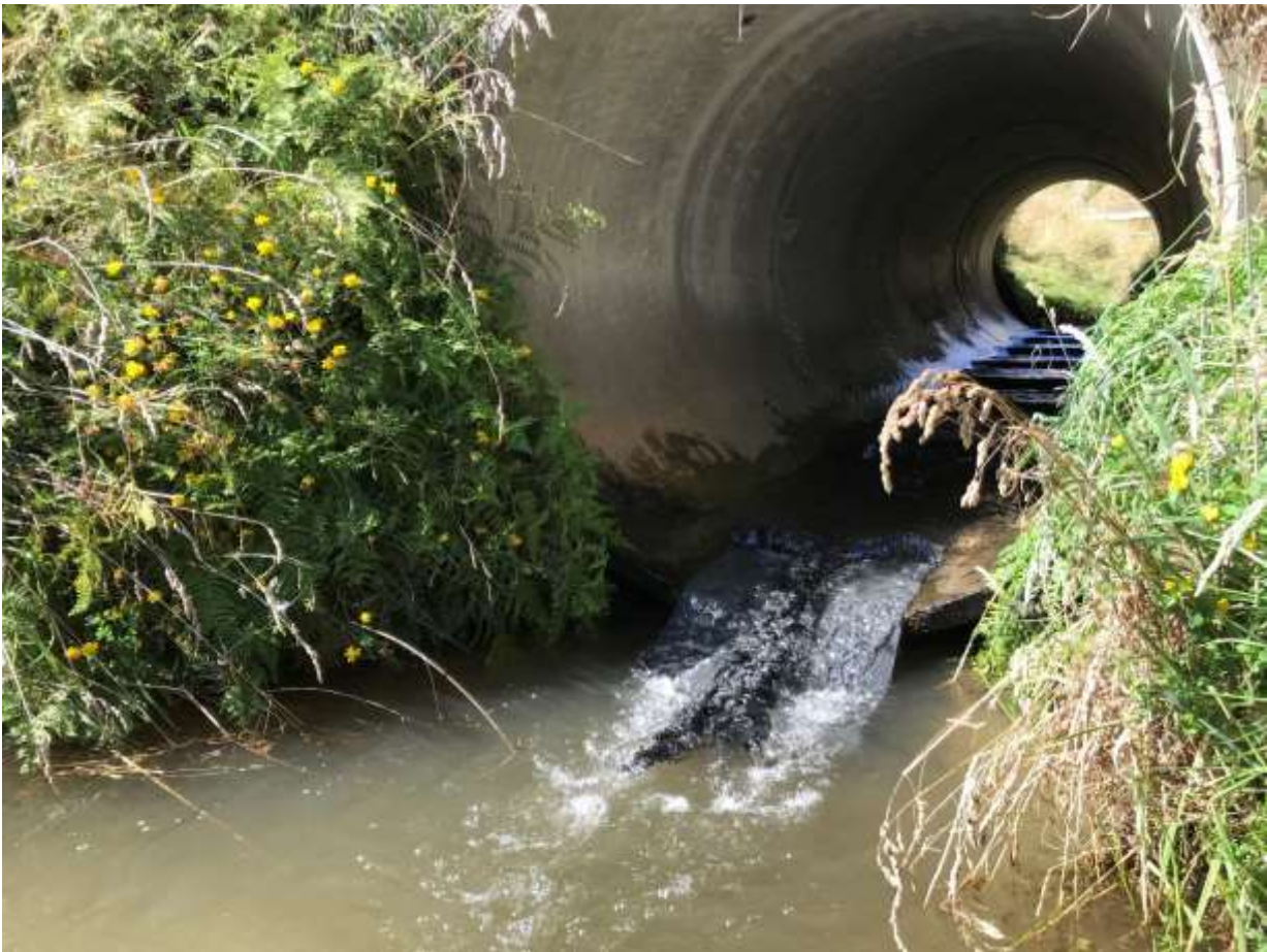
Figure 16: This culvert in the Waoku Stream catchment, a sub-catchment to the Koputaroa, had a small perch. This was remedied by placement of rubber matting and mussel rope.
