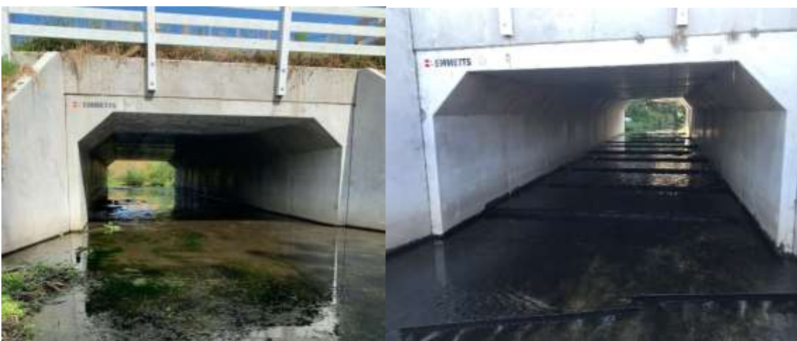
Figure 7: Left: Large box culvert located in the Awarua Stream, Whanganui, prior to remediation. Right: Remediated culvert with lengths of flexi-baffles and a fish ramp installed.
