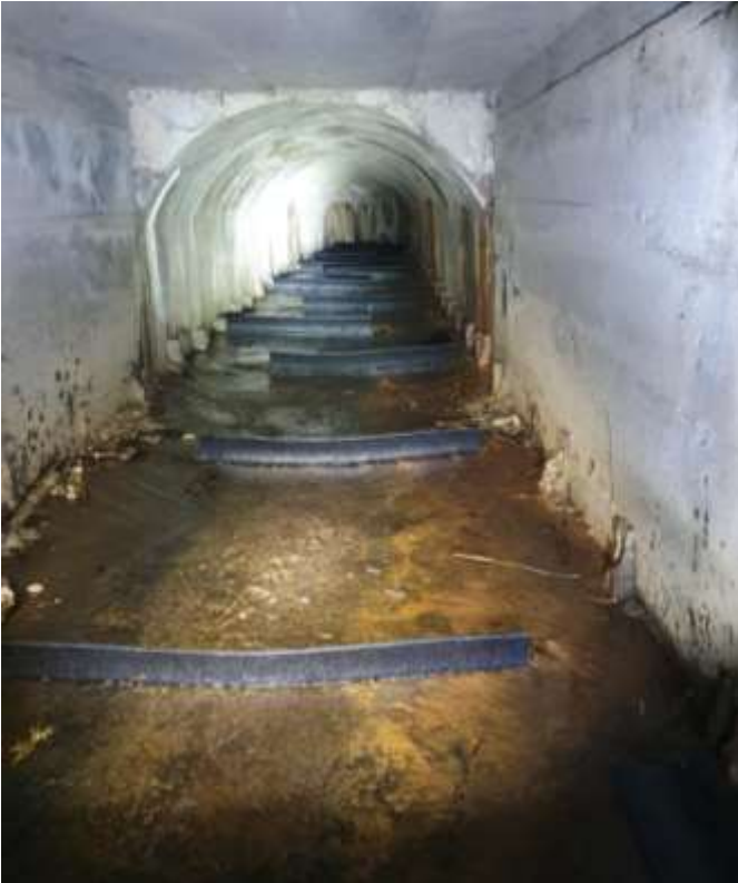
Figure 8: Culvert remediation, Purua Stream, Whanganui. Flexi-baffles were installed throughout this 195 metre culvert running under SH4 into the Whanganui River.
