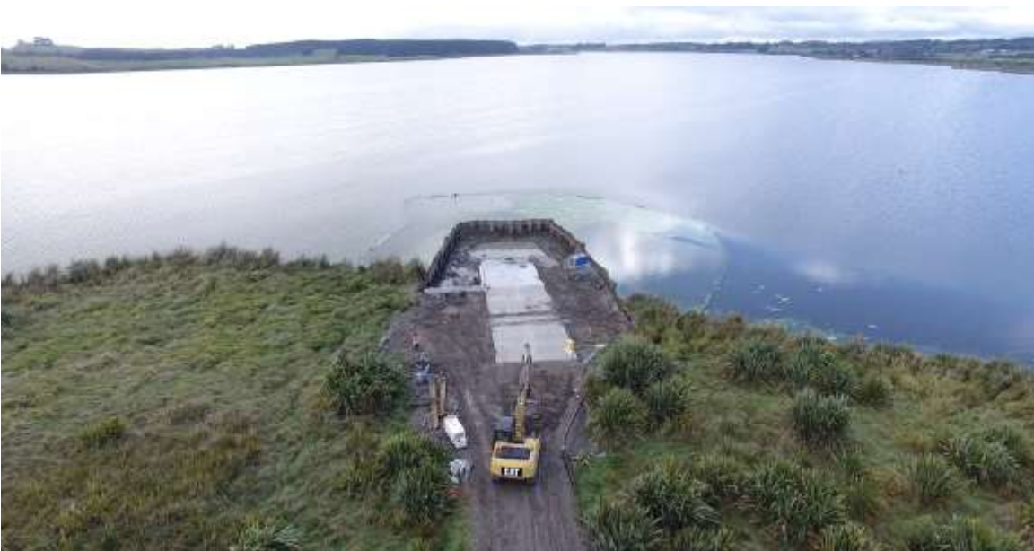
Figure 20 The Lake Horowhenua boat ramp prior to the removal of the sheet piling and sediment curtain.
