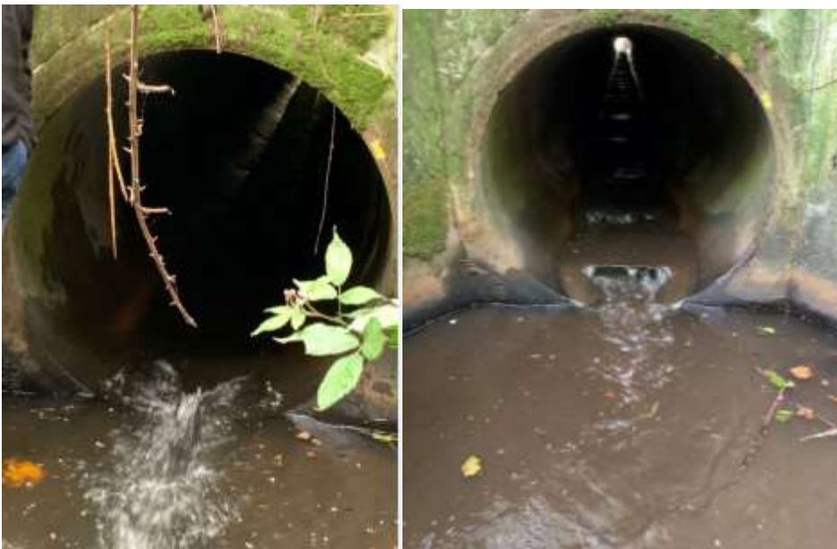
Figure 6: Culvert remediations in a tributary of the Mangawhero Stream, Ohakune. Flexi-baffles were installed throughout with mussel rope (top right) attached to the apron of one culvert to allow climbing species to pass.
